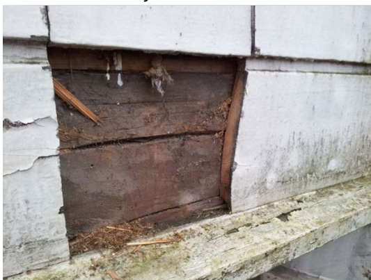
Picture 5. Wooden materials in bad shape
