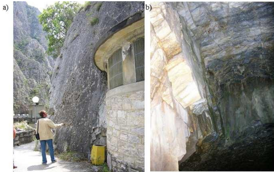
Figure 2. a) A look of the Rock Masses at the zone of future pre-cut; b) a look inside the excavation
