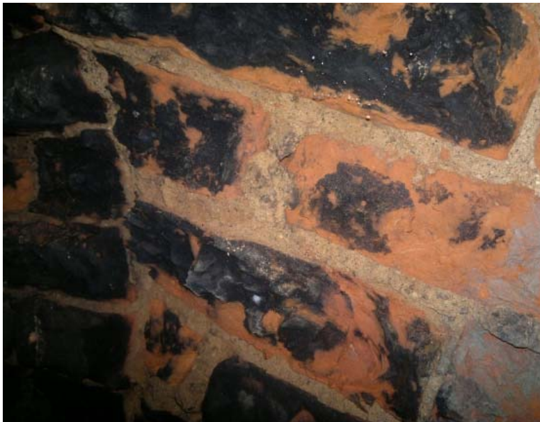
Figure 3. The result of the breaking opening of support area of the vault
