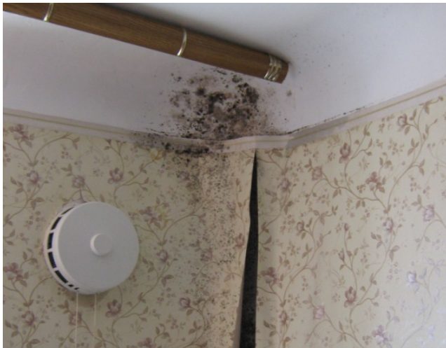
Figure 5. Mold on the internal surface of the internal and external walls joint in the living-room
