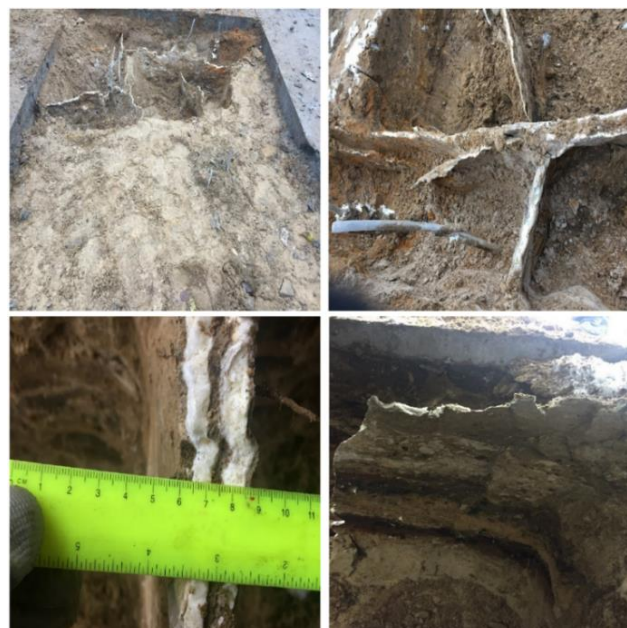
Figure 1. The distribution patterns of the resin propagation, which formed in the massive of the sandy soil after the injection process [1].
