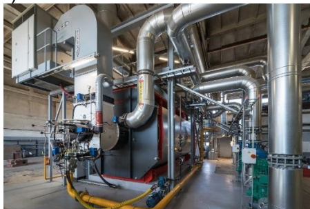
Figure 5. Hot-water boiler “BOSCH UT M-64”.
