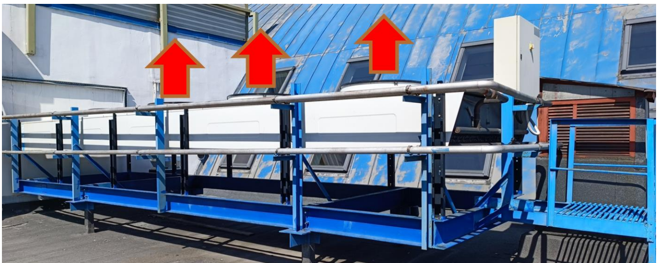
Fig. 2 – Air condenser ECA12N9P10C2, manufactured by FRIGA-BOHN, France (photo taken by the author)
