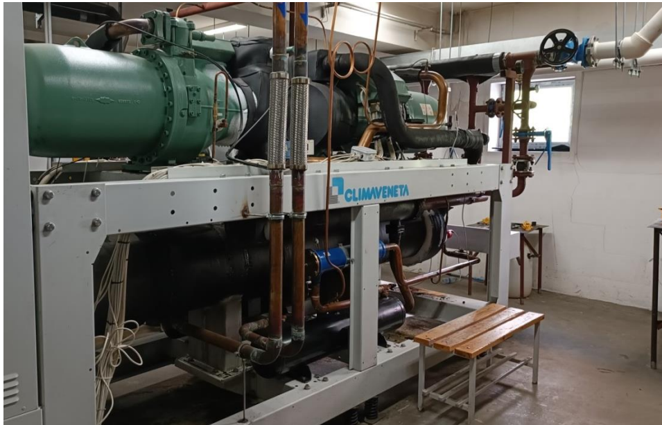
Fig. 1 – Evaporator-compressor unit Climaveneta BE/SMED-BT (photo taken by the author)
