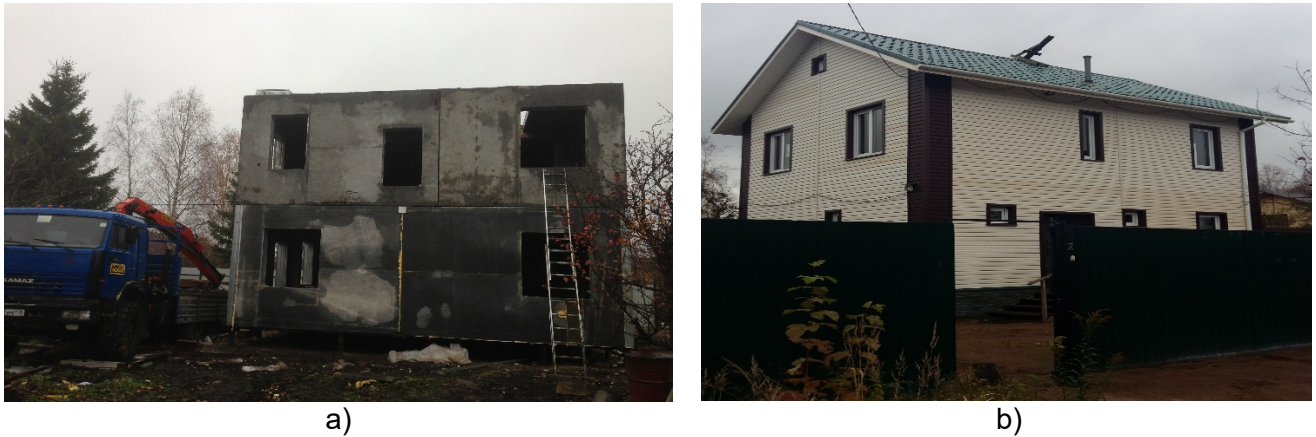
Fig. 1 – a) The mounted panels of a LSBK house on the 5th day of construction b) The finished house on the 15th day of construction
