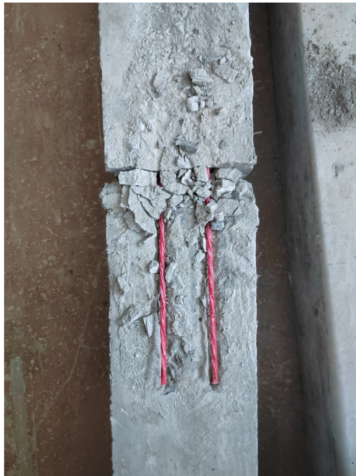
Рис. 10 - Разрушение соединения (вид на арматуру) Fig. 10 - Destruction of the connection (view of the reinforcement) Image by the author of the article
