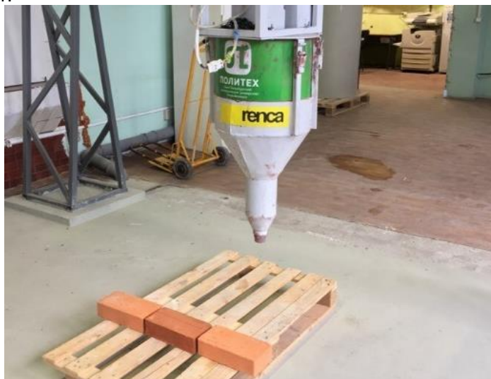
Picture. 10. A row of masonry before feeding the solution with a 3D printer
