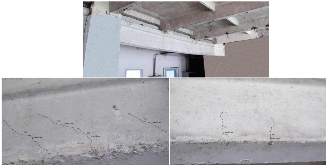
Figure 4. General view and characteristic defects of the evaluated precast beam and ribed slabs
